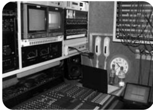
Inside one of the mobile control units
