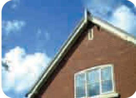
Modern design of window without rebating that does not blend well with older properties
