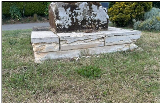
Plate 4: Failed Clipsham Stone
